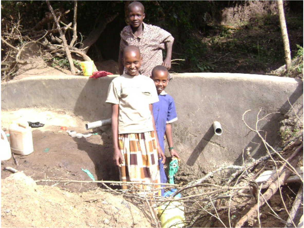
Oloitiko spring weir and the off take pipes from where the community will be drawing the water once the protection of the spring is completed. The girls have come to draw the water which now flows from one of the off take pipes. This spring will provide portable water to Oloitiko community throughout the year.
